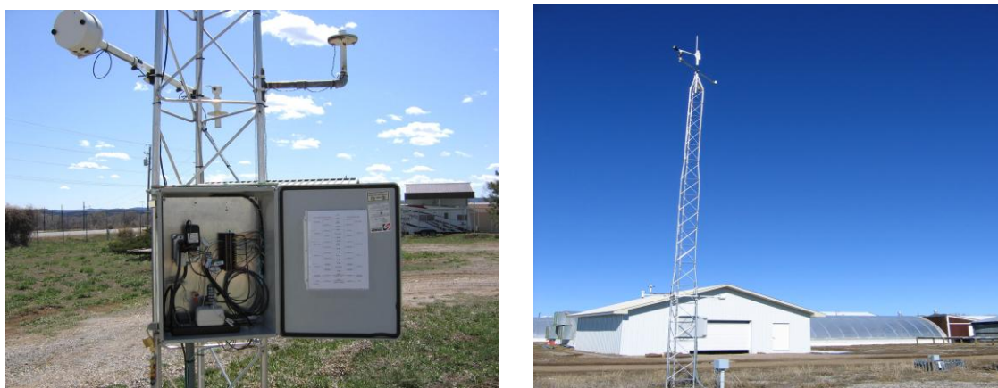
Figure 3 – Ute 1. Meteorological tower and weather resistant, surge protected enclosure box (left). The thirty-foot meteorological tower (right).
